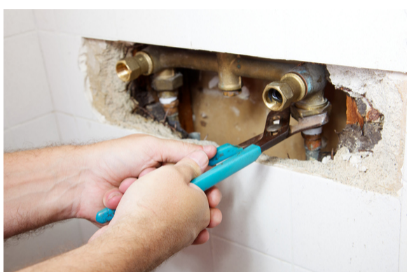
Leaky pipes can be costly.
